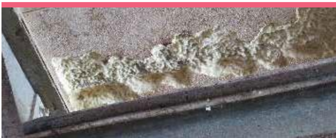
Figure 4. Damage to insulation caused by rats.
