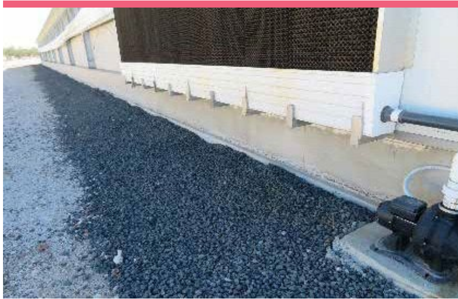
Figure 2. An example of compacted road base along shed parameters to prevent rodents burrowing.
