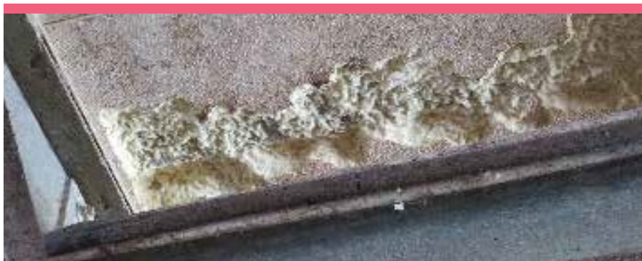
Figure 4. Damage to insulation caused by rats.
