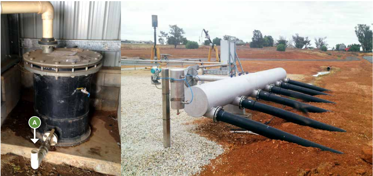
FIGURE 3 Above-ground condensate collection drums (“knock-out pots”) at Australian piggeries.
