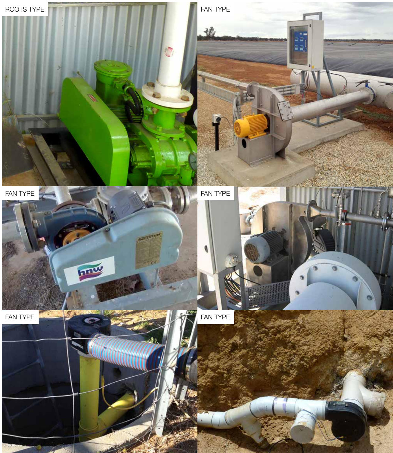
FIGURE 1 Various biogas blowers at Australian piggeries. Blowers boost the pressure of biogas so that it can flow via subsequent pipelines and treatment vessels to the biogas appliance. Often there are condensate collection drums in the pipeline before the blower to protect the blower from entrained moisture droplets.
