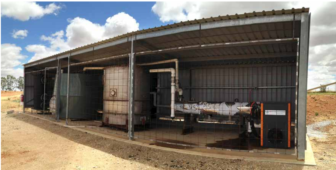
FIGURE Biogas treatment infrastructure at Case Study 6 piggery
