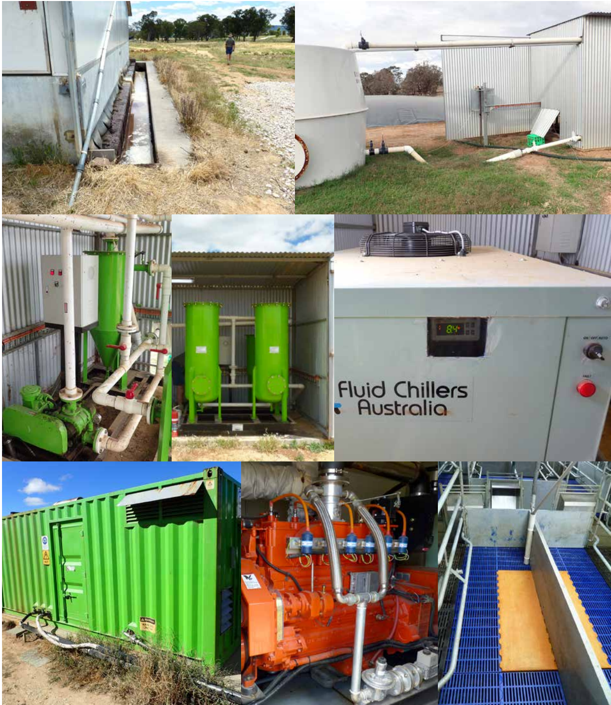
FIGURE Biogas equipment at Case Study 1 piggery
