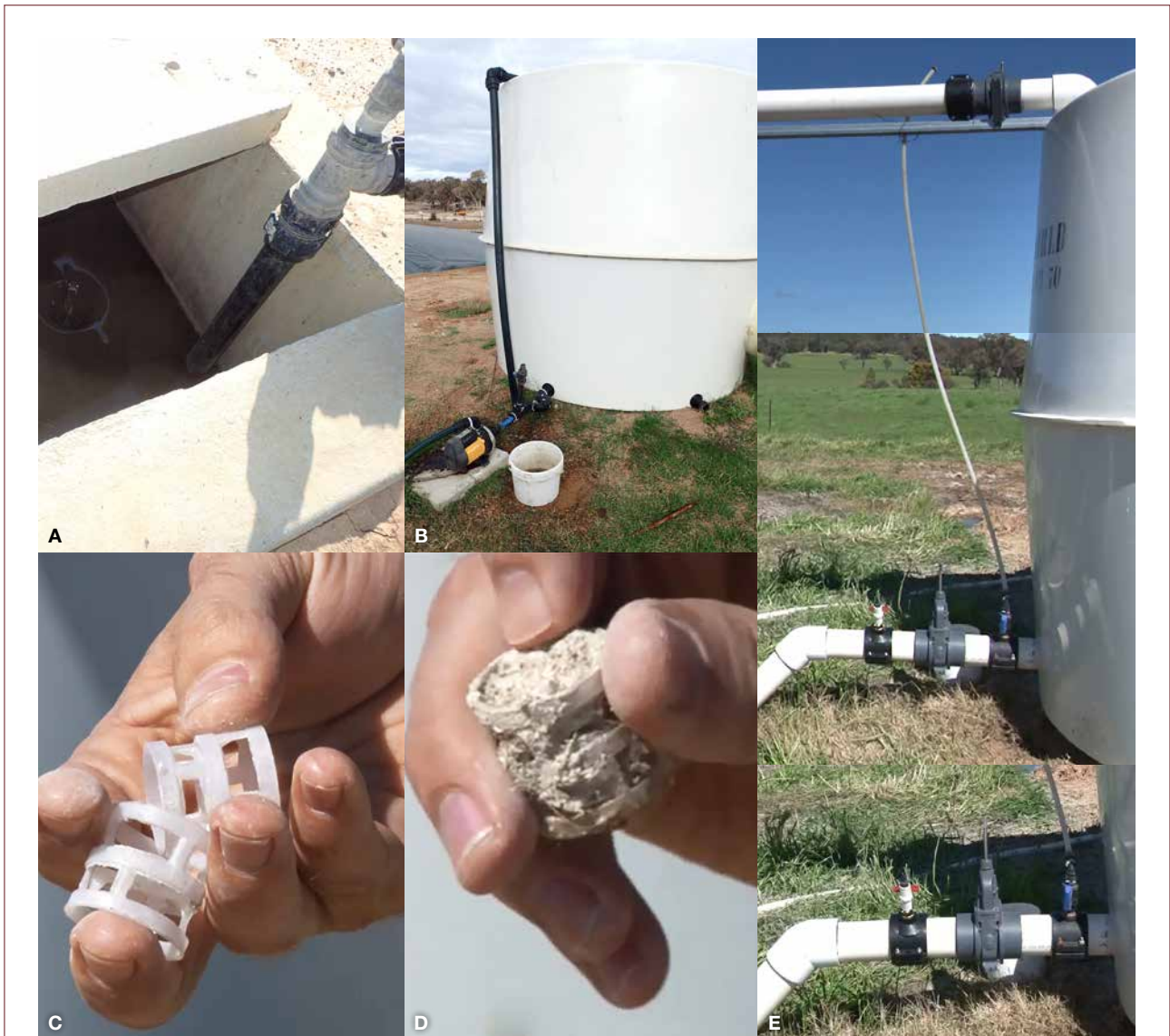
FIGURE Biogas infrastructure at Case Study 4 piggery
