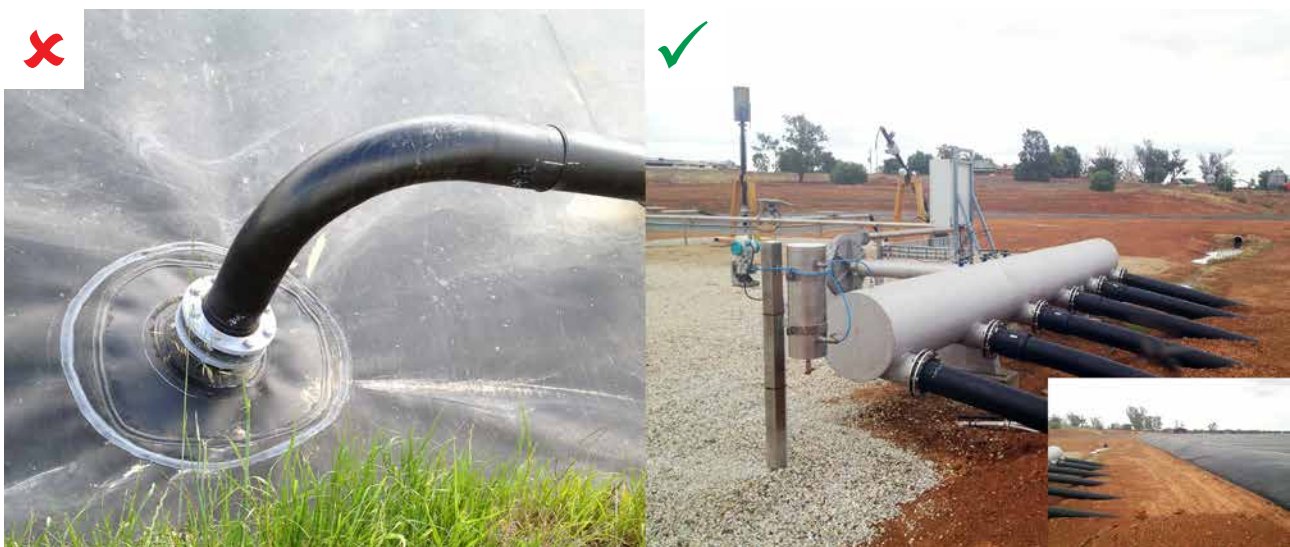
FIGURE 6 It is preferred for pipework to protrude through the pond bank (right), because then pipes and joints do NOT move up and down when the cover becomes inflated to store biogas. When biogas pipework is connected directly to the cover (left), the joint with the cover can fail prematurely, which is unwanted. Similarly, excessive movement along other cover joints and pipe joints can impose unwanted stresses and increase the potential for premature failure.
