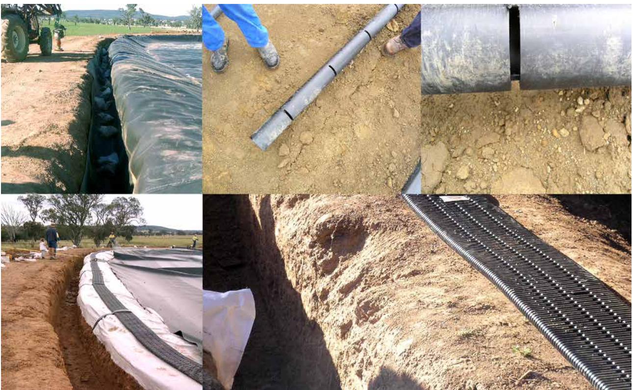
FIGURE 5 Biogas collection pipework under the cover at Australian piggeries, which can be either slotted pipes with burs removed, or more commonly perforated HDPE flat panels. The perforated panel HDPE has been preferred because it is easily secured and does not move or roll with movement of the cover.
