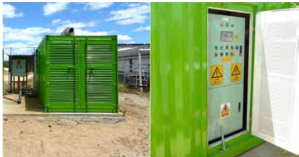
FIGURE 6 Guarded electrical supply with warning signage on a shipping container with a biogas-fired generator inside. Also note the illuminated emergency switches which are located outside the shipping container.
