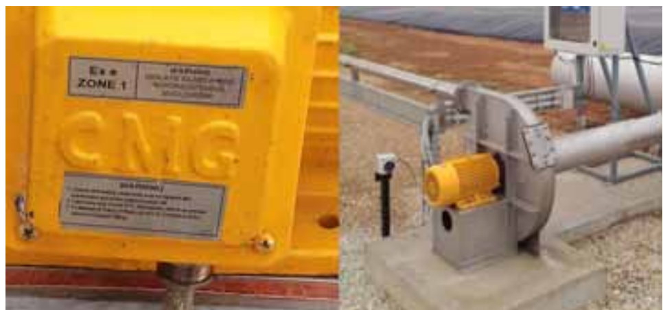
FIGURE 2 Example of a biogas fan blower at an Australian piggery rated to Zone 1 in accordance with AS/NZS 60079.10.1: Classification of hazardous areas – explosive gas atmospheres .
