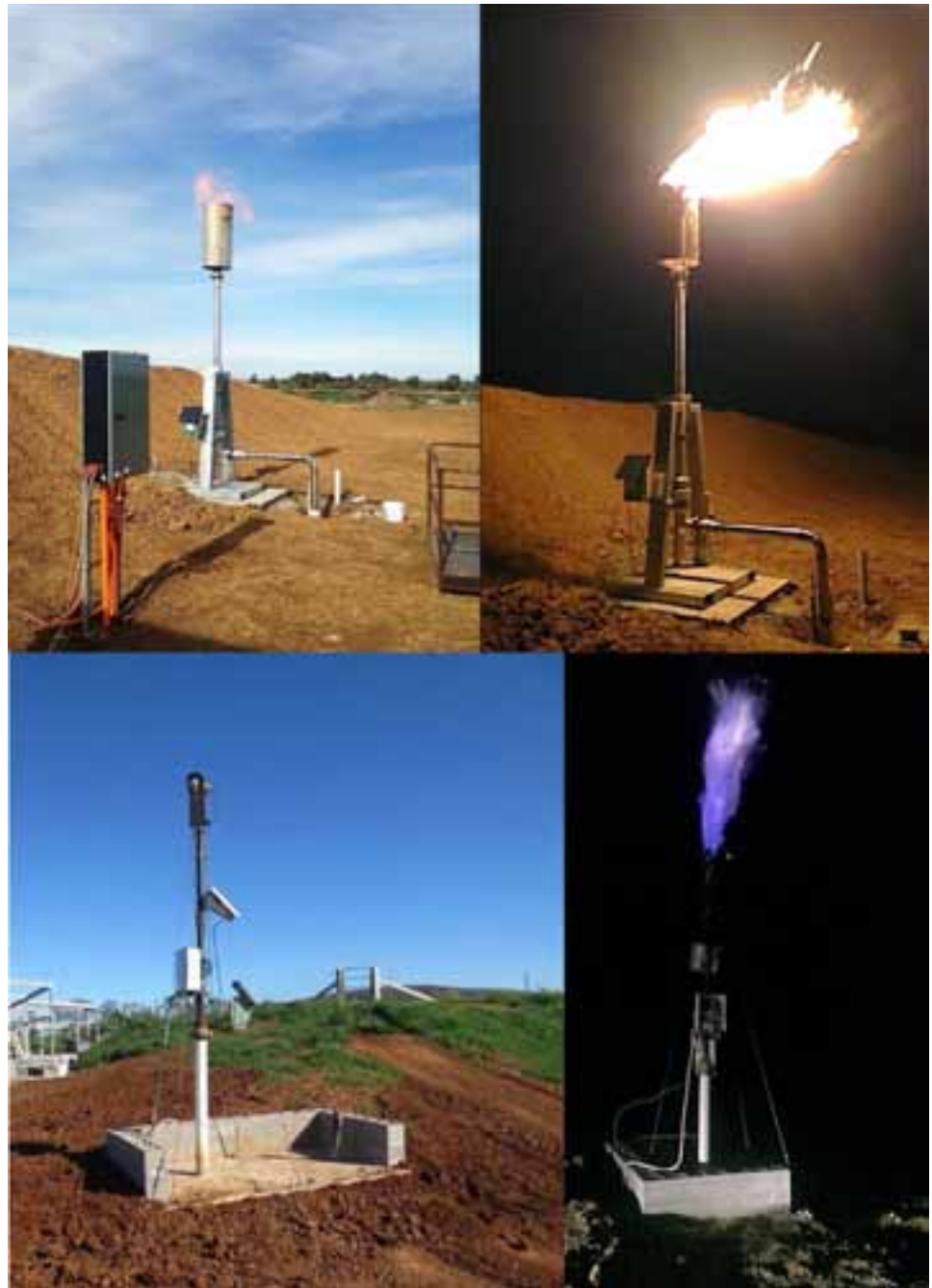
FIGURE 1 Biogas flares at a piggery in Australia. Note the shrouding on the top of some of the flares, which can provide some protection and may reduce fire risk. Note also that vegetation has been cleared around the flare to reduce fire risk.
