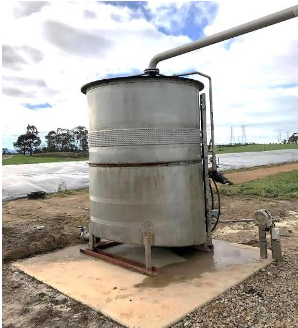
Figure 3 External scrubber tank used for removal of H 2 S. Effluent is pumped to the top of the tank via the pipeline with in-line strainer visible on the right side of the tank. A small quantity of air is continuously injected into the scrubber tank by the air blower visible to the right of the tank. The covered pond and biogas inlet pipe are visible at the back and base of the tank. Note how the electrical supply for the air pump is set-back at a nominal distance away from the biogas piping and scrubber tank, to exclude viable ignition source from where elevated methane concentrations may exist due to potentially leakages. This was by expert design of an external consultant.
