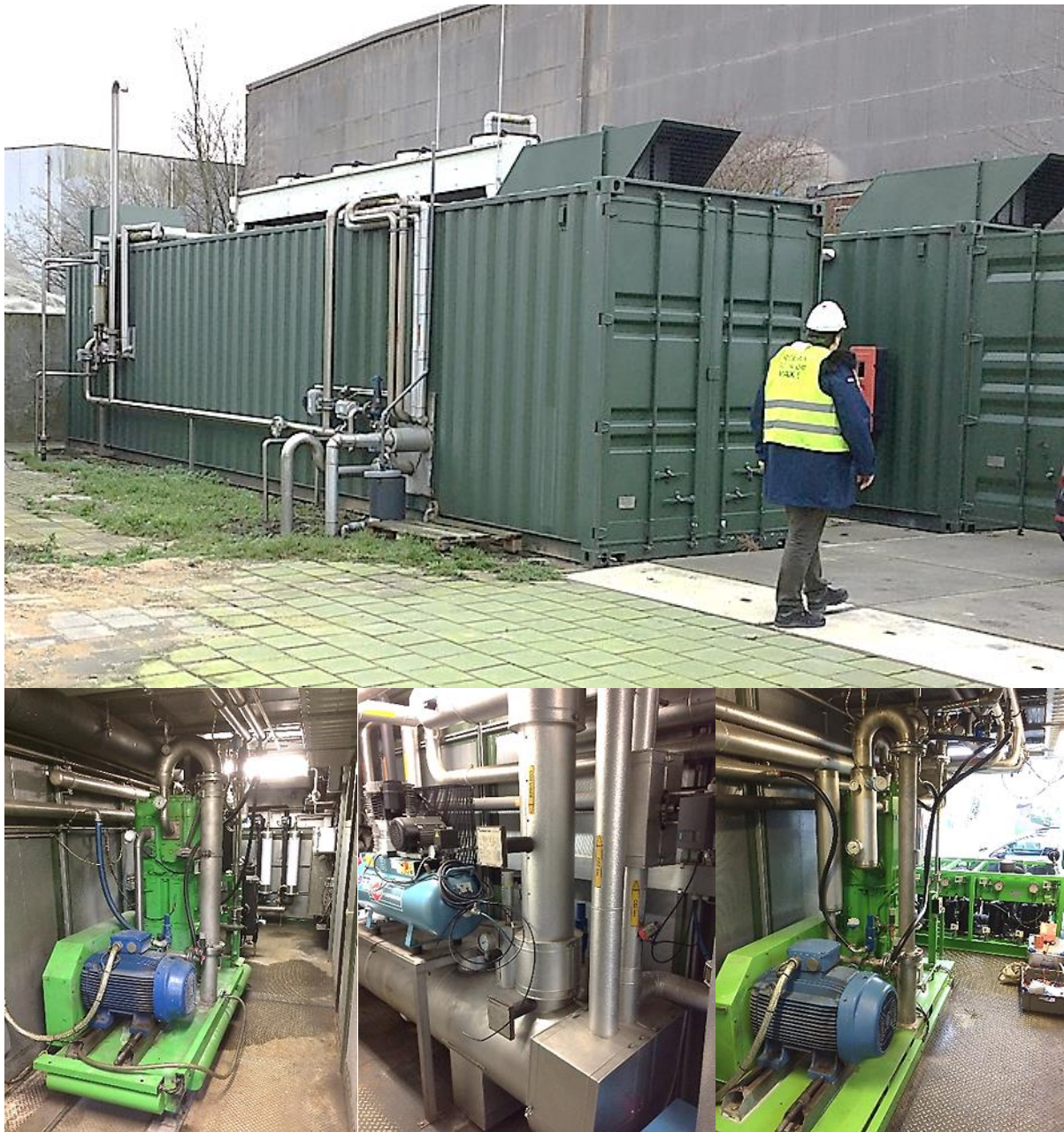
Figure 14 Example membrane-based biogas upgrading infrastructure in the Netherlands, by Pentair Haffmans. The infrastructure is fully containerised inside pre-assembled 40-foot containers, making it modular and readily transportable. Photos also show infrastructure inside the containers, including a compressor and membrane units for separation of methane from CO 2 (left), heat exchangers (middle), and refrigeration units able to produce liquid CO 2 . This example system is identical in size to what would be suitable for the large piggery concept, i.e. 250 m 3 .hr -1 raw biogas flow. Source: Tait (2018).
