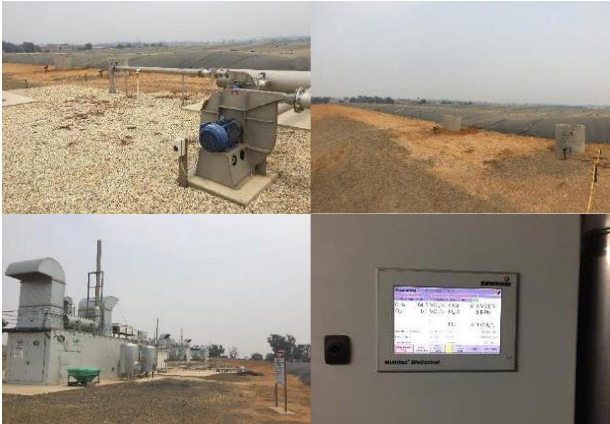
Figure 11 Photographs of biogas infrastructure, taken during the project site visit. The infrastructure includes two covered anaerobic ponds (top) and three 500 kWe Evo 2G generators (bottom left corner), producing electricity with biogas containing about 65% methane (bottom right corner).
