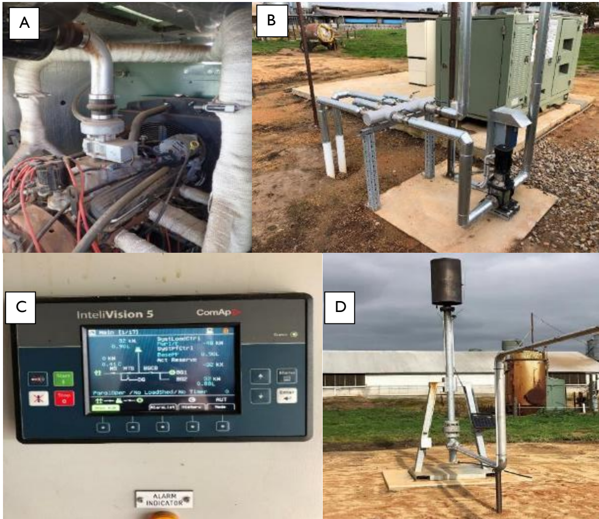
Figure 5 Photos of the biogas-fuelled combined heat and power engine generator (A, B, C) and the emergency flare (D). The respective photos show (A) the generator unit when originally purchased second-hand with wear and tear due to disuse and (B) after retrofitting and installation at the case study piggery, (C) the control system screen, and (D) the solar-spark partially shrouded emergency flare. The flare has a thermocouple to confirm whether the flare is operational by measuring the presence of a hot flame.
