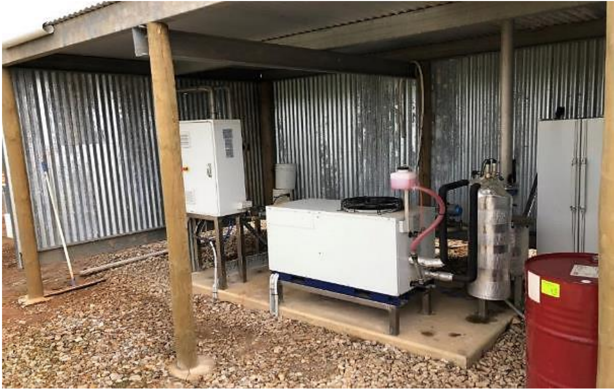
Figure 4 Electrical chiller (not absorption chiller) and shell and tube heat exchanger used to condense and remove moisture from the biogas prior to use at the case study piggery.
