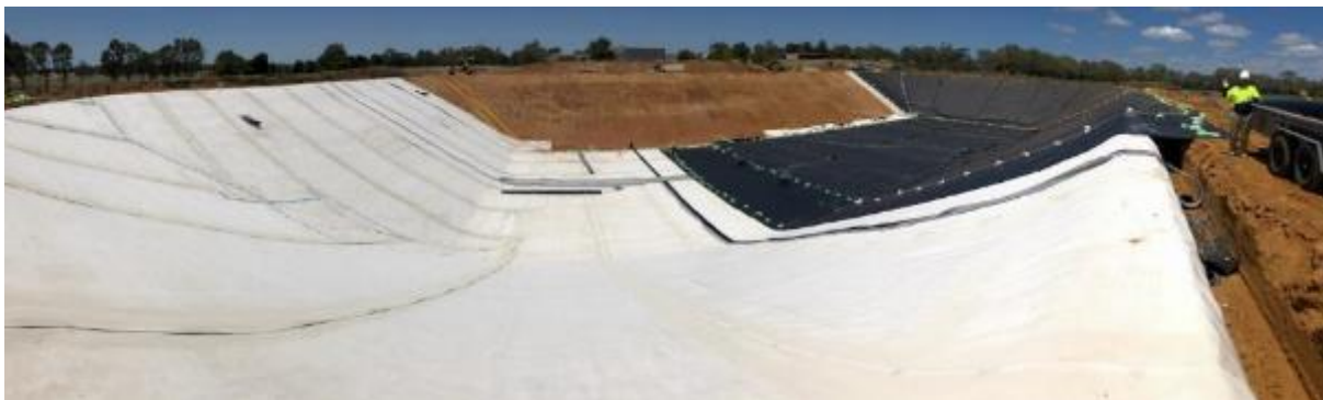
Figure 7 Example in-ground dam lining performed by Waterlogic, showing liner on the left and geotextile protective layers (Source: Waterlogic).
