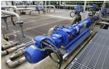
Figure 10: Installed Mono 'EZ strip' progressing cavity pump
