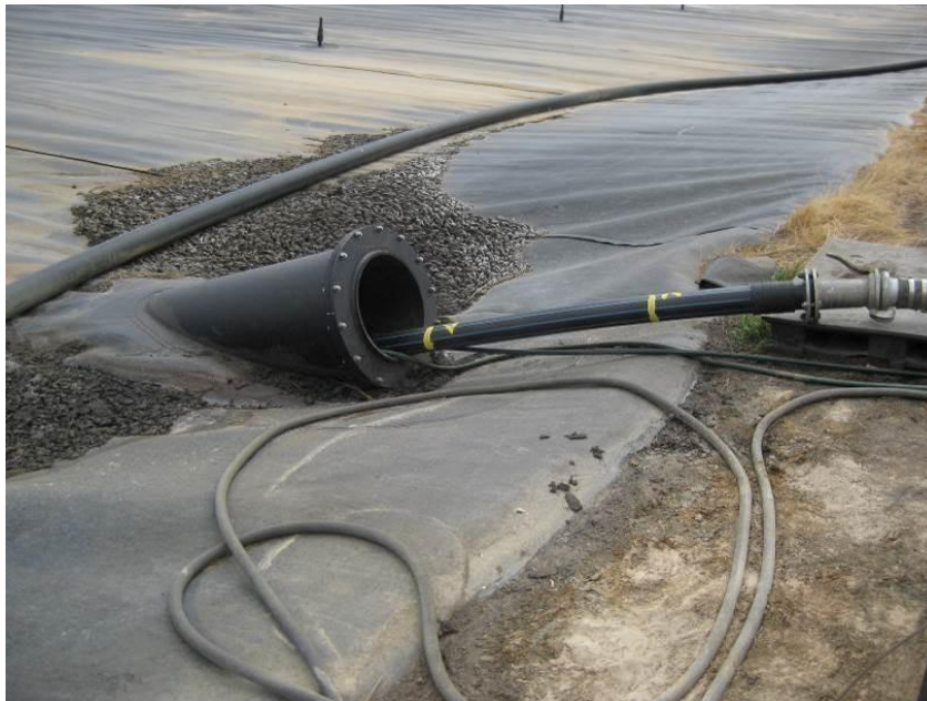
Photograph 40: Suction pipe inserted into CAP
