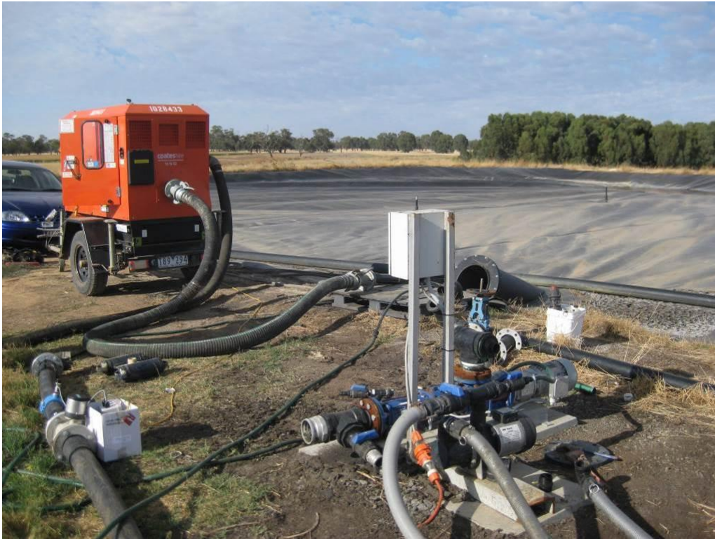
Photograph 42: Vacuum pump and pipework
