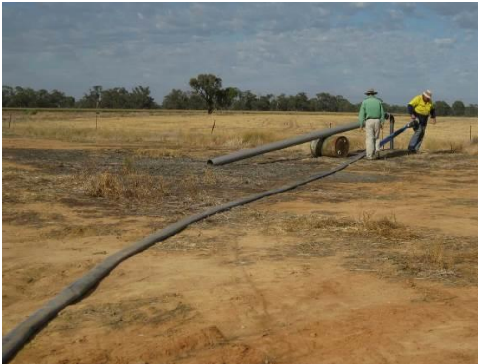
Photograph 28: Piggery A slurry pipeline riser adjacent to drying bays
