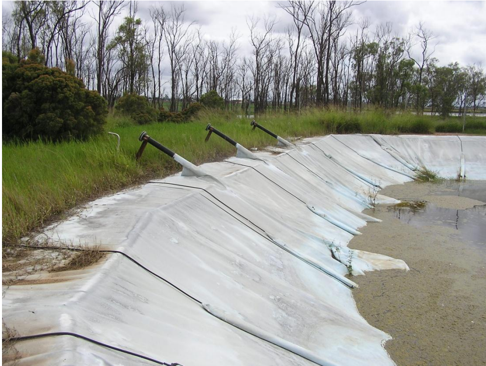
Photograph 16: Sludge extraction pipelines (deflated pond cover)
