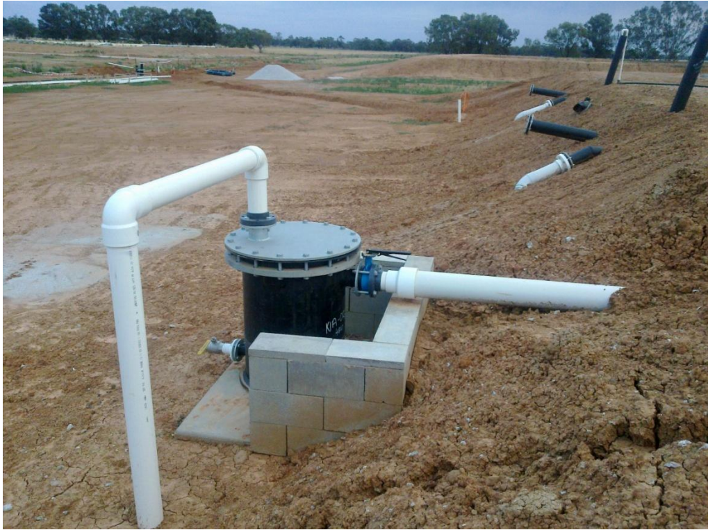
Photograph 18: Sludge (black) and effluent (white) removal pipes
