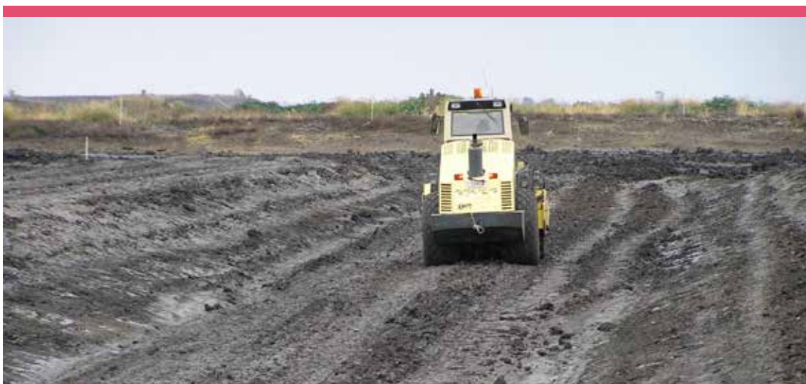
Photograph 6 Vibrating pad foot roller compacting the base of a SEPS channel (photo courtesy of Alan Skerman)
