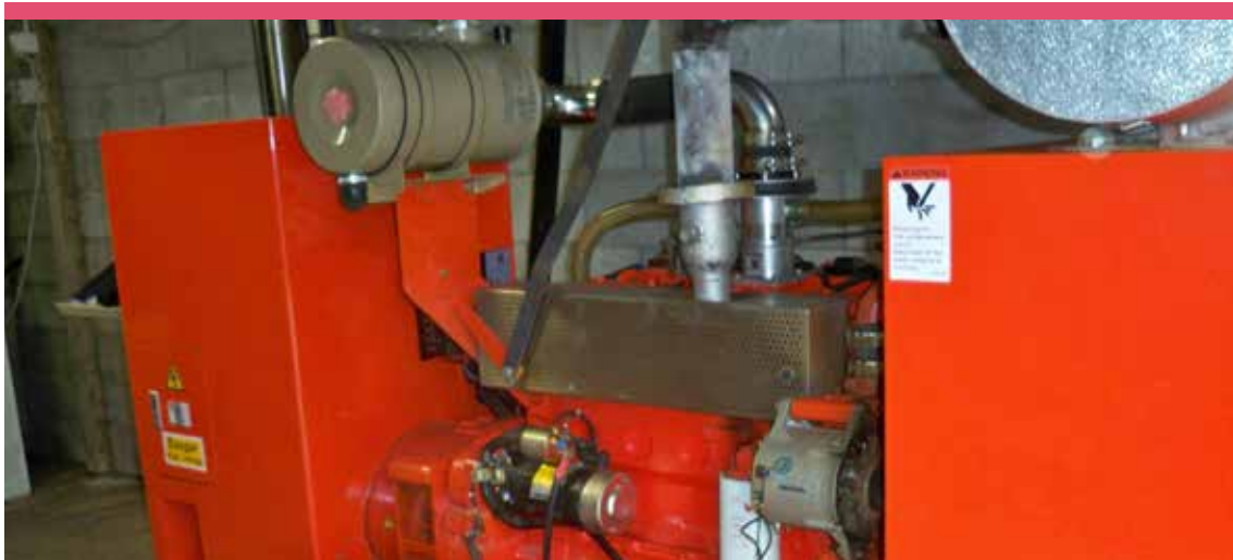
Photograph 10 Combined Heat and Power Generator
