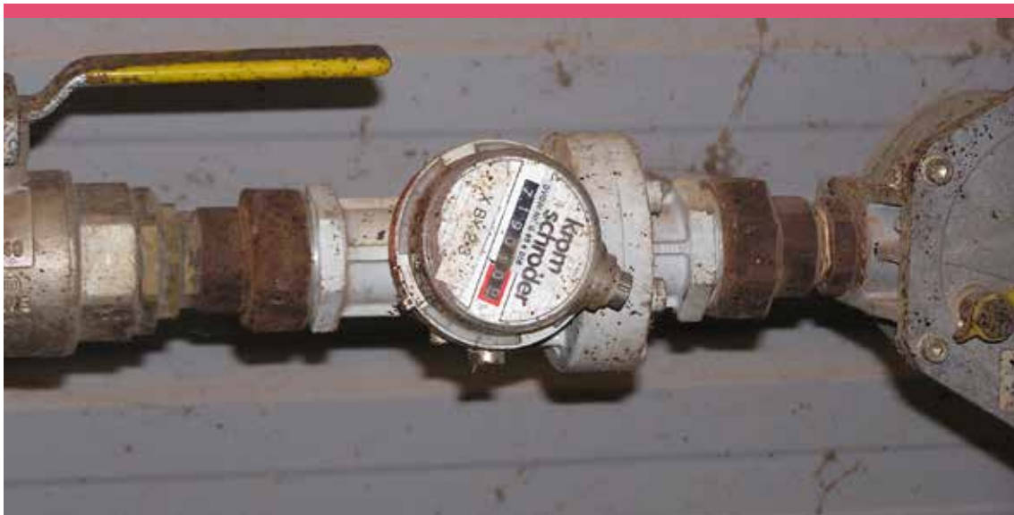
Photograph 7 In-line Gas Meter
