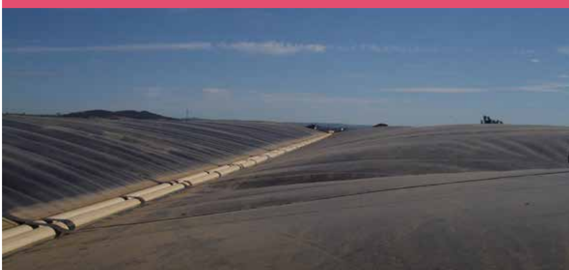
Photograph 9 Covered Anaerobic Pond at a Piggery
