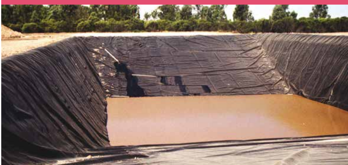
Photo 3 Plastic lined trapezoidal pond with steep batters on long sides and flatter batters on ends
