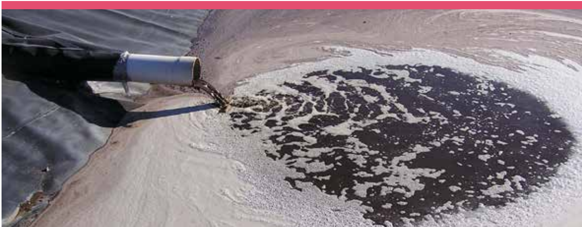
Photograph 4 Effluent pond inlet pipe discharging above top water level
