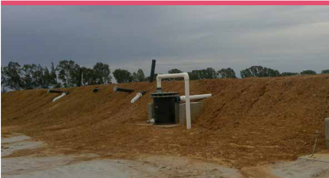
Photograph 6 Sludge extraction ports being installed along outer wall of new CAP (Photo courtesy of Tom Smith)
