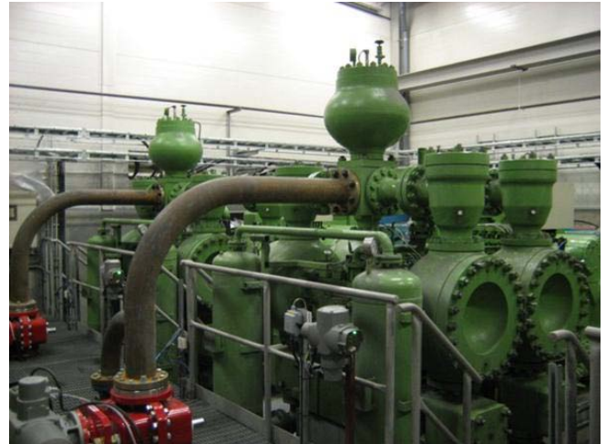
Figure 4 – Heavy duty industrial GEHO PD - ZPM Pump
