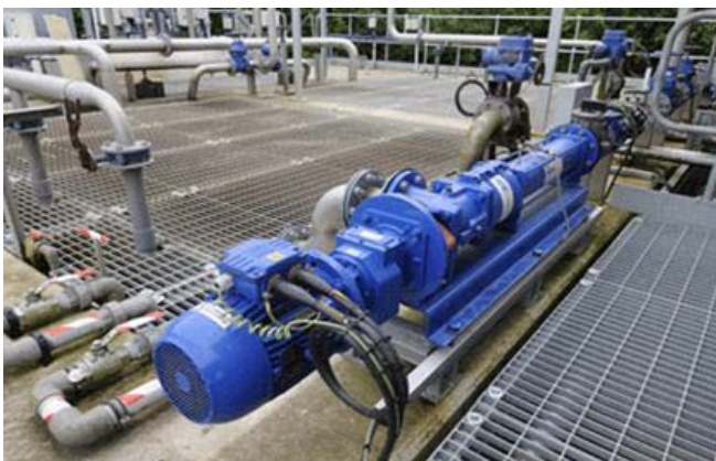
Figure 10 – Installed Mono 'EZ strip' progressing cavity pump
